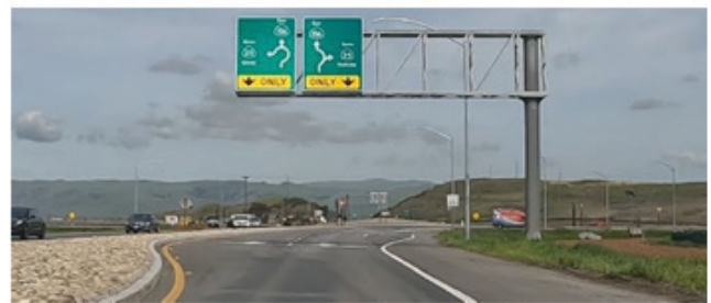
Figure 3. Configuration of Overhead Signs Installed at the Rotor Turbo.
