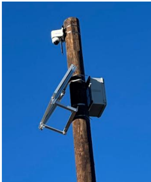
Solar-powered pole-mounted deployment
