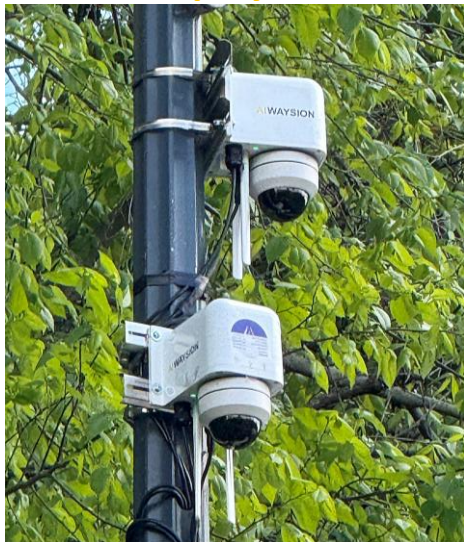
Grid-powered pole-mounted deployment
