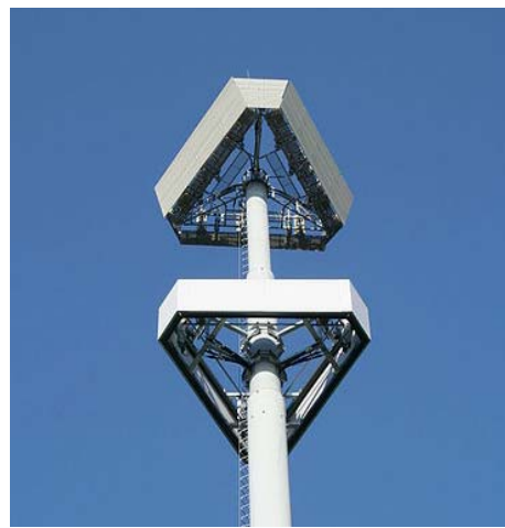
Figure 1 - Cell Tower Example 2
