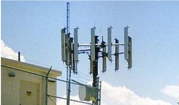
Figure 2 - Cell Tower Example 1
